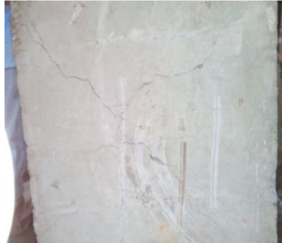
Figure 2: Crack patterns while testing the slabs
