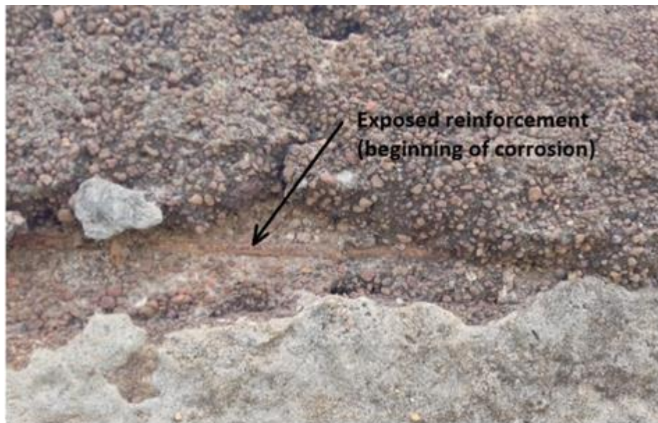
Figure 12: Dissolution and erosion of the material expose the reinforcement bars of the Founkama micro-dam dam (Photo. Babilas Hountondji, 2026).
