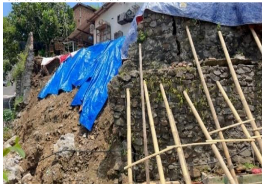
Figure 2. The presence of a soil retaining wall at the site of the landslide
