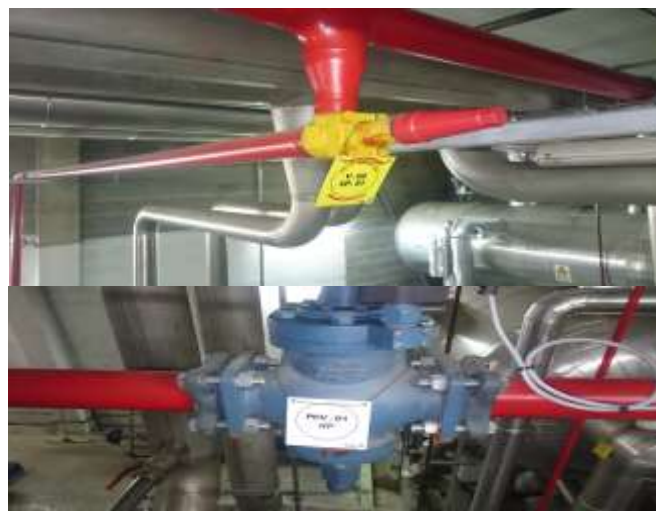
Figures: Two of the valves causing additional pressure drops
