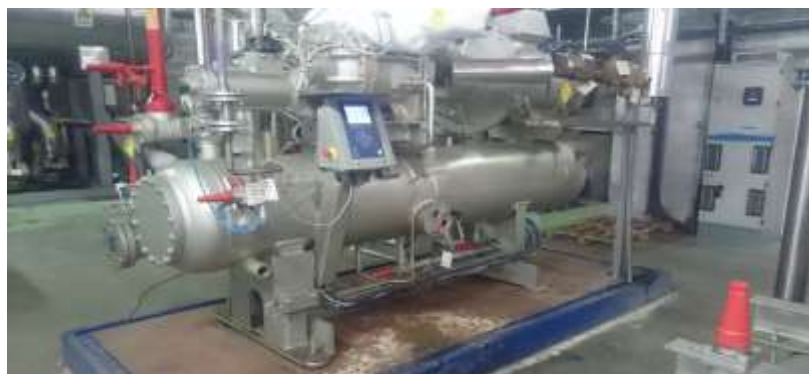
Figure 3: Front view of one of the three screw compressors
